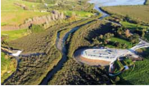
Matakohe East End - works adjacent to Matakohe River Bridge No.2 on May 3
